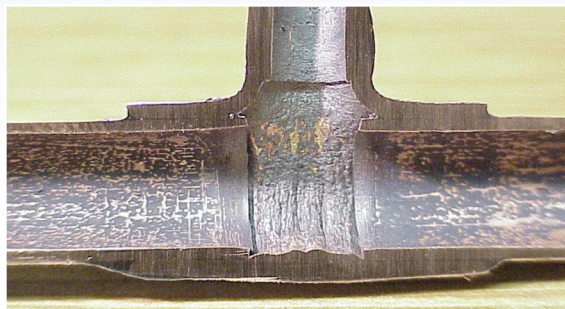
Copper tubing brazed without nitrogen purge. Notice the black oxide deposits.
