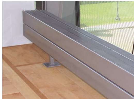
Curtain Wall Convectector on Pedestals
