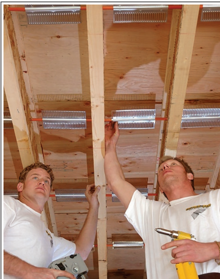
Ultra-Fin Radiant Floor Heating System installed from below
